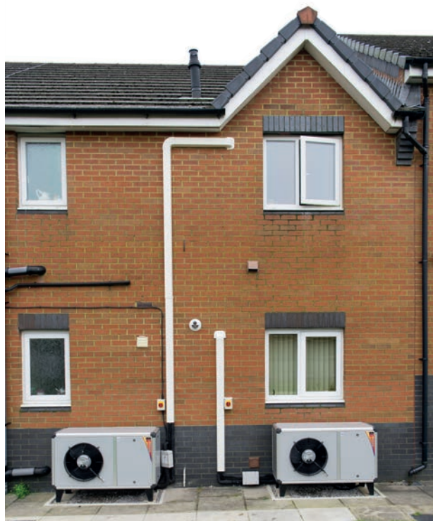
Two air source heat pumps connected to homes in the Bridgend trial
